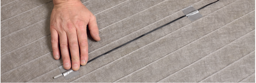
FIGURE 2.16: Secure floor sensor probe
